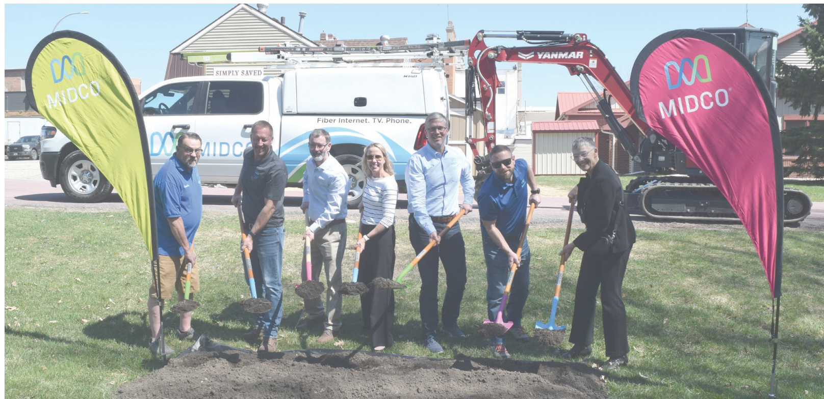
Midco is starting to break ground and install fiber cable all around Janesville. On Thursday, April 16, they held a ceremony at Veterans Memorial Park, which included council member Ivan Maas (far left), City Administrator Clinton Rogers (center left), and County Commissioner DeAnne Malterer (first to the right). (Photos by Michael Roy)
